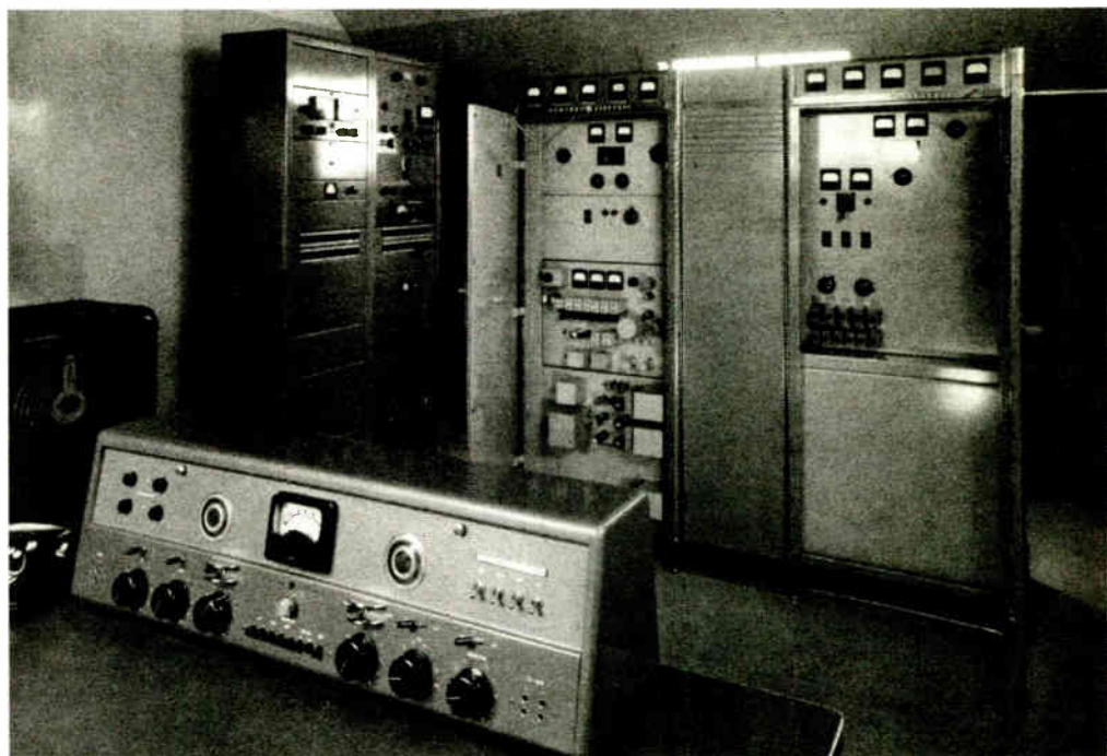
Late 1940s WFBL(FM) in Syracuse sports a GE Phasitron FM transmitter, with 250 watt exciter at left and 3 kW amplifier at right. Stations were manned by First Phone operators, hence the console. WFBL was in a Quonset hut; notice the curved wall. Steve Auyer, from whose collection this image is taken, said the station went on in 1947 but failed to make money and the owner returned the license three years later. It is now WNTQ.
