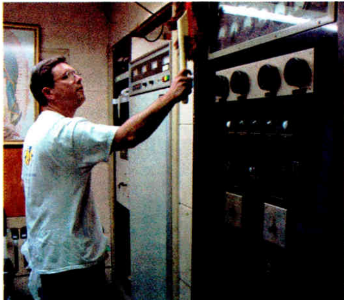
KWG, Stockton. That's engineer Paul Shinn dusting the 1930 transmitter.
