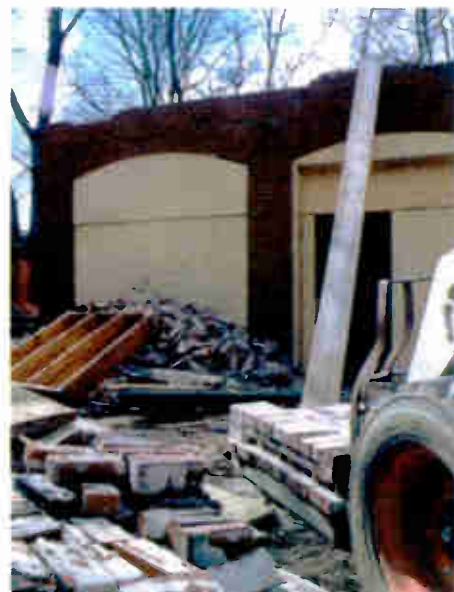
The demolition of Frank Conrad's garage in Wilksburg, Pa., the original 8MK/KDKA, in March 2001.
