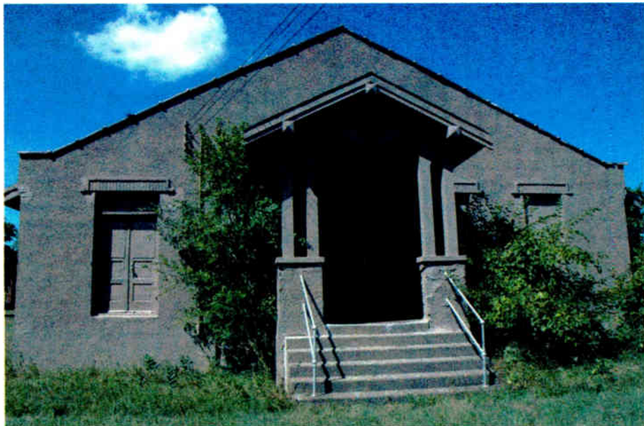
WCCO's original 1924 transmitter building, constructed at the Coon Rapids site for the 'superpower' 5 kW signal, still sits on a corner of the property and is used now for storage.
