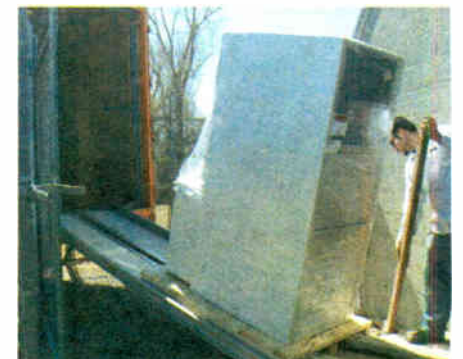
Steve Moore maneuvers a new Harris Z16 transmitter into KRPS(FM).
