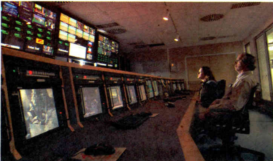
The Network Operations Center is the heart of AFN. Operators in Mannheim and at a similar facility in Vicenza, Italy monitor the signals and manage the insertion of European-interest spots and news for 40 radio and 10 TV channels.
