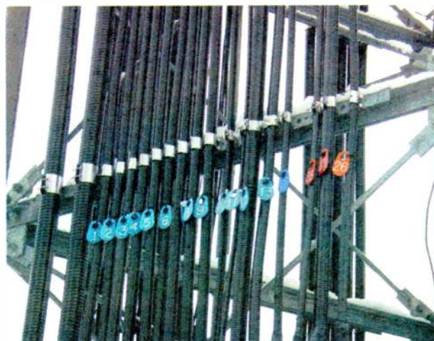
Fig. 2: Tagging coax lines makes identification easier.
