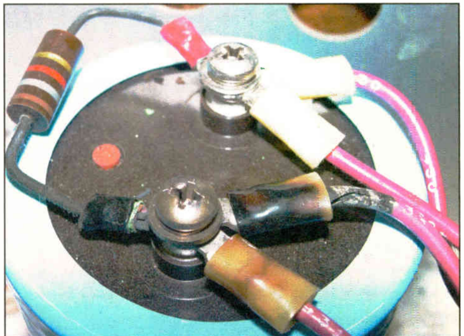
Fig. 2: A bright light can help you discover pending failures like this overheated terminal.
