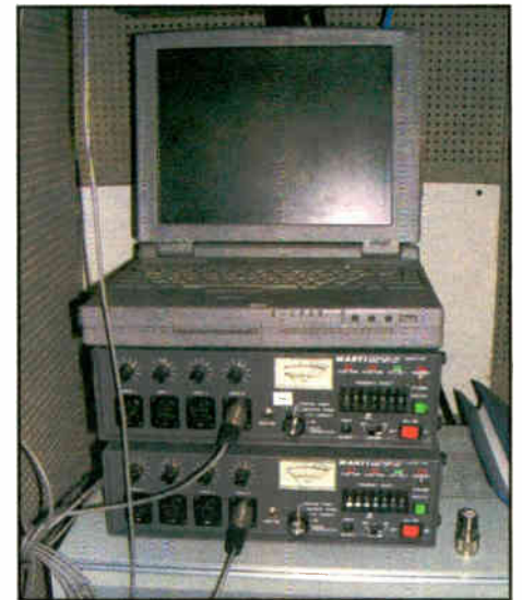
Marti backup transmitters and Moseley LAN link are used to extend the Dalet network.
