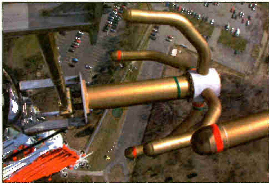
Part of the Lynx antenna, mounted on the tower.
