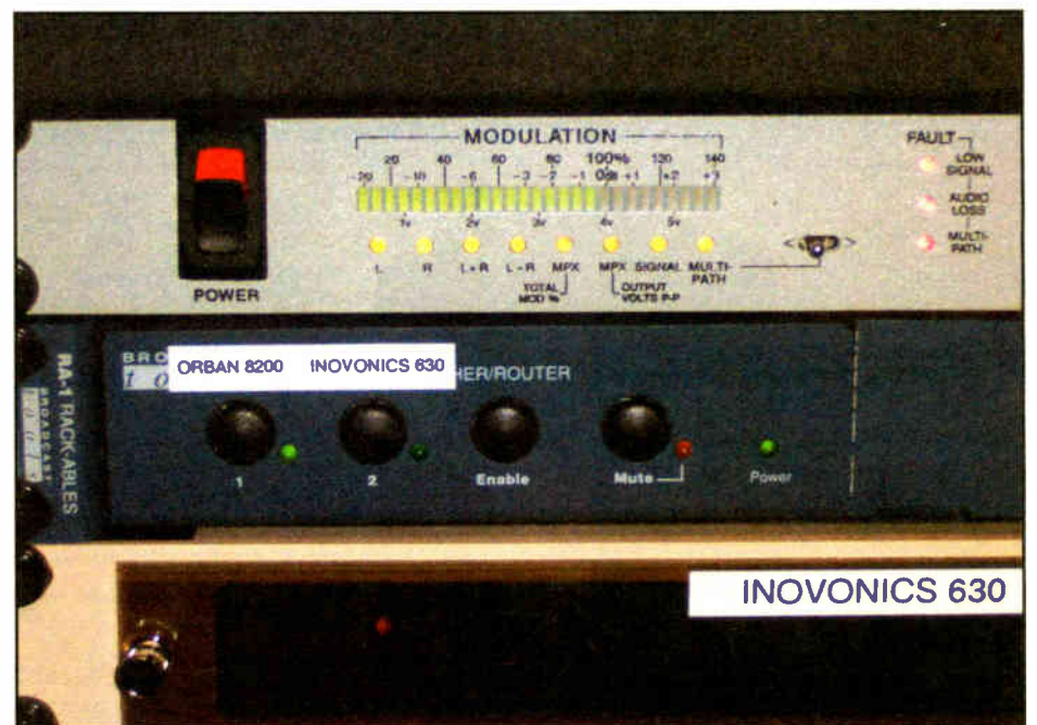
Closer front view of switcher showing the normal operating mode in this configuration.
