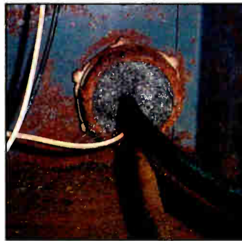
Fig. 3: Plug all holes and wire pass-throughs with steel wool.
