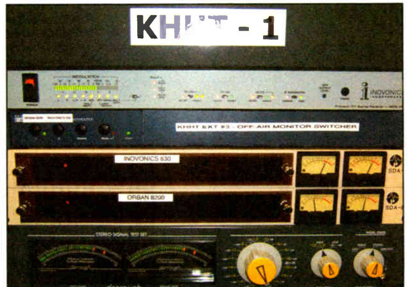
Front view of racks displaying switcher in position #1, which is the normal Orban 8200 processed audio feed.
