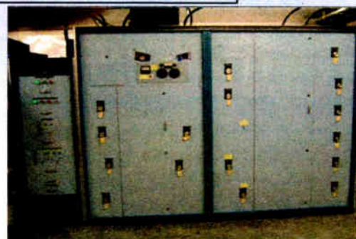
Kintronic Phasor Cabinet/Control Rack Installed At KNWC-AM 5/2.3kW 1270kHz Five Tower DA-2
