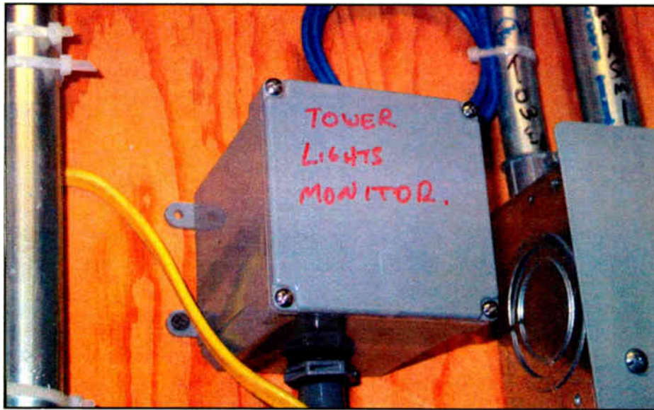
Enclosure holds the control that monitors tower light power.
