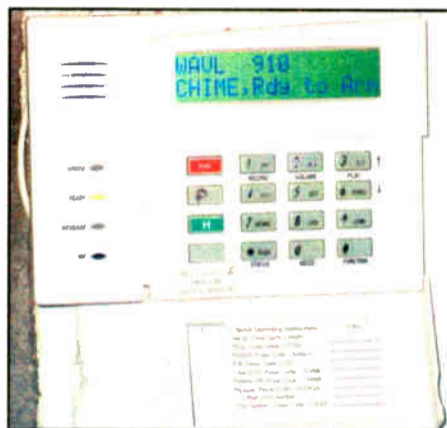
Control keypad for the system has voice capabilities and announces what is going on in the alarm.
