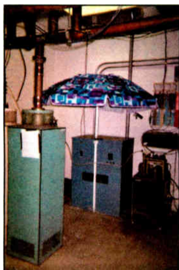
Fig. 1: An umbrella was pressed into service to keep the high-voltage vault dry.
