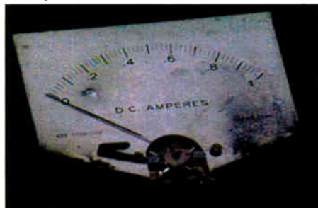
Fig. 1: Check the location of meters in the circuit before touching them.
