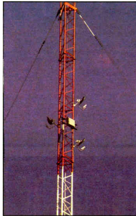
The Motorola Canopy cluster, including NEMA enclosure, was installed on KLZ's east tower.
