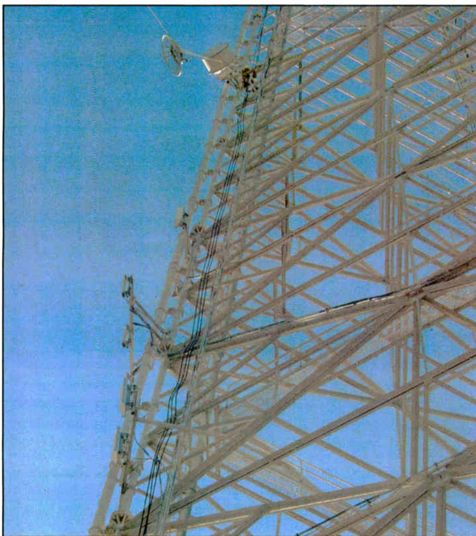
Fig. 1: The 7/8-inch lines running up the left side were lashed to the leg with steel wire. Winds tore the cables from their mounts.
