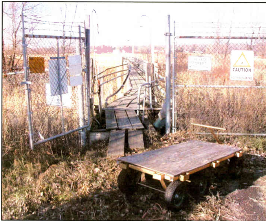
A 1,000-foot catwalk and cart were used to transport the Kintronic 'sectional' phasor to KSTP's Tower Two building.
