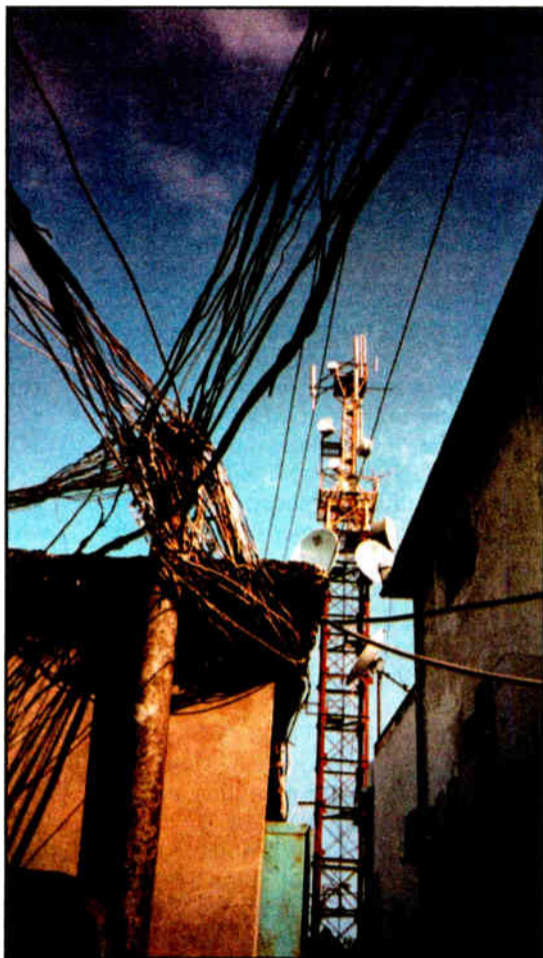
A nest of wires is visible outside the broadcast communications center in Poti, Georgian Republic.
