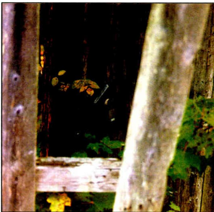
Fig. 3: The lock was locked, Mr. FCC Inspector! Too bad the fence gate rotted around the hasp.
