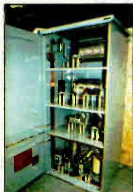
AM Triplexer Cabinet 3 x 2.5kw
