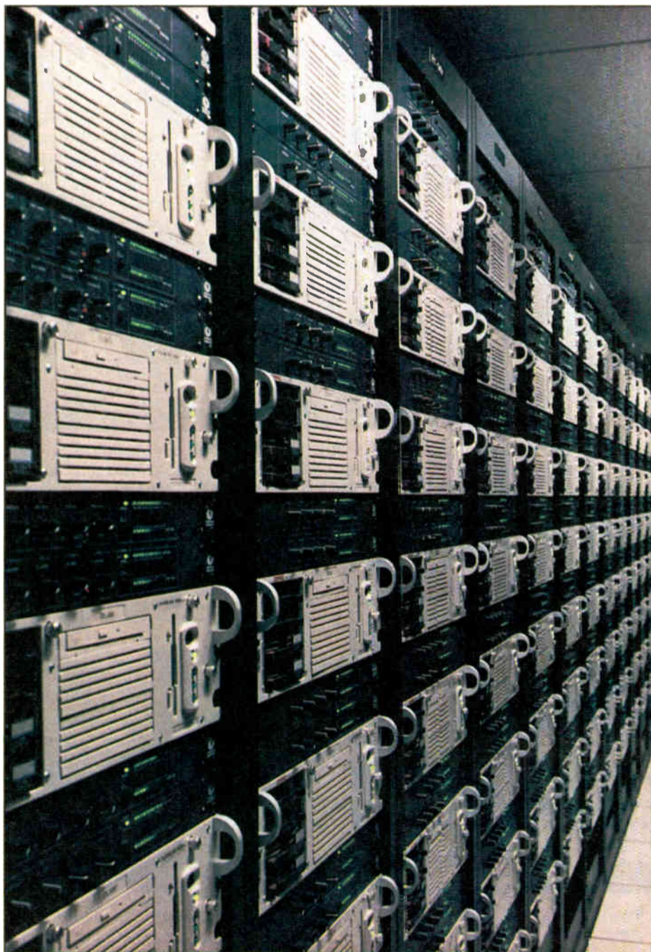
Compaq Proliant encoding stations line a wall in 'Grand Central.'
