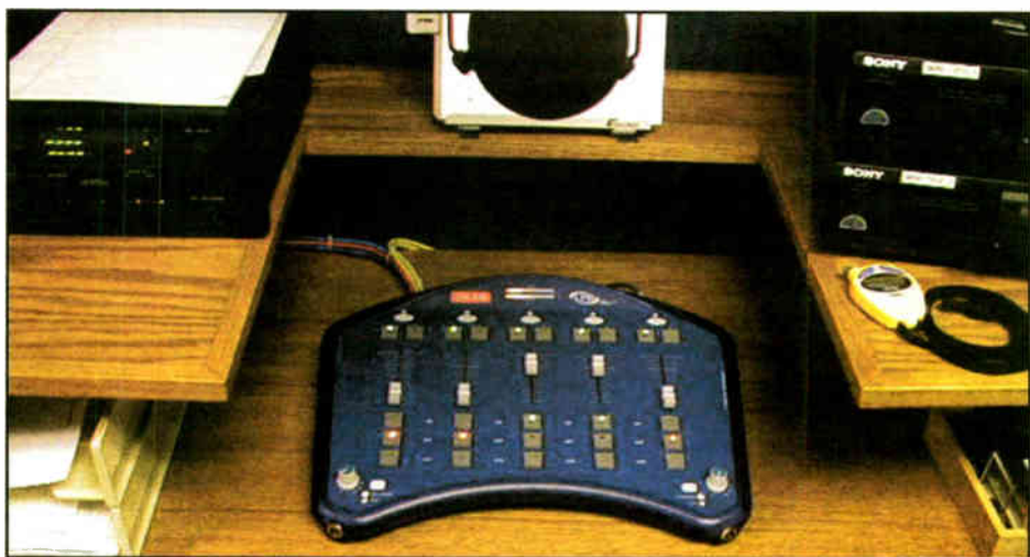
The LPB Blue 5C console was installed recently at 100 kW WHPE(FM), High Point, N.C., a Bible Broadcasting Network station using Blue for on-air and production.
