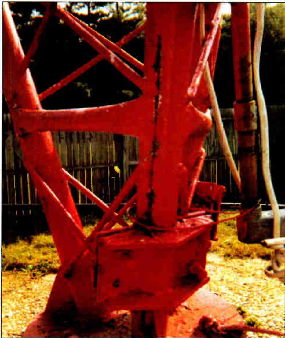
Fig. 1: Hollow tower legs can split.
