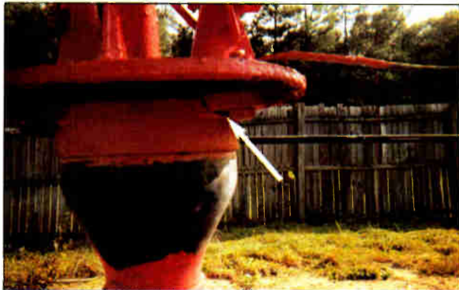
Fig. 2: The arrow indicates a cracked bracket
