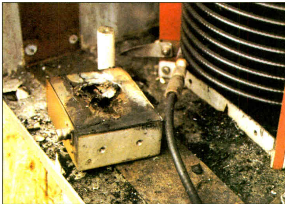
Fig. 2: Inside an ATU, lightning has damaged a sampling toroid.
