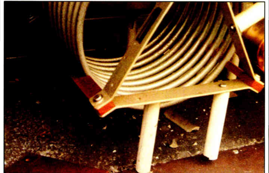
Fig. 3: Check for cracked or broken insulators supporting coils and other components in an ATU.
