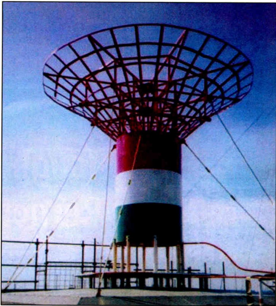
San Remo, Italy CFA installation
