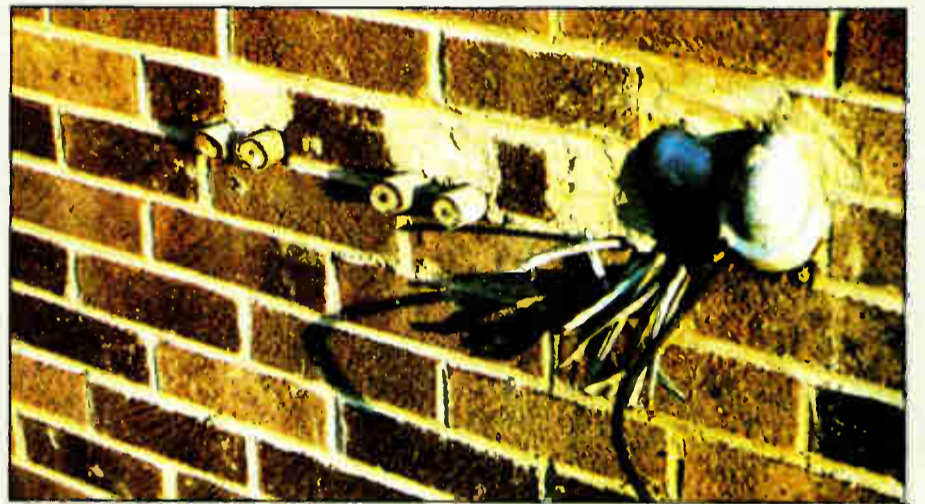
Figure 3: Supervise contractors to avoid accidents like this!
