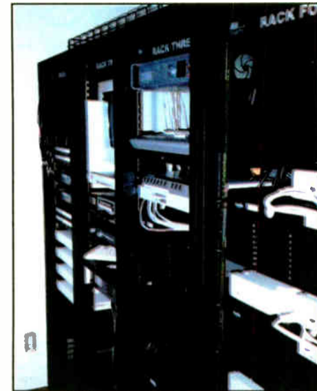
In the Rack Room
