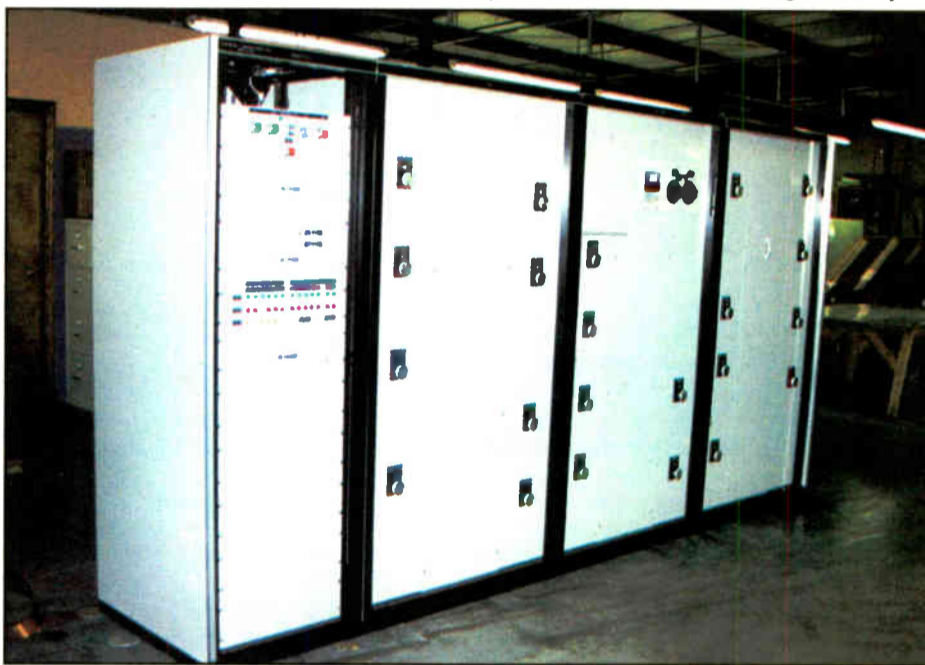
Kintronic Custom-Built AM Transmitter
