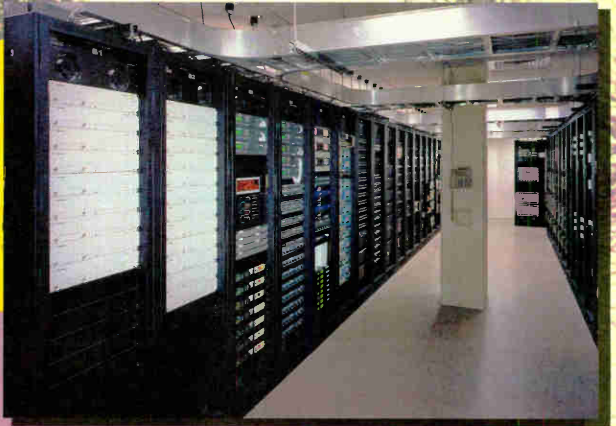
Main Rack Room containing 46 racks of equipment
