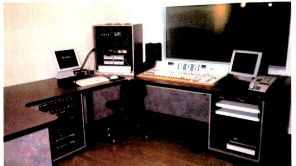
Control Room A
