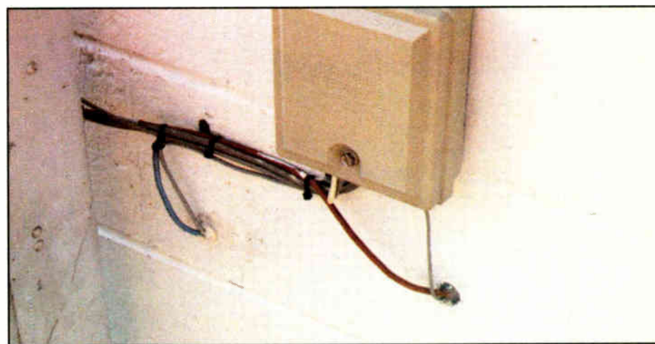
Figure 4: Rubber caulk can be removed to make way for future cables. In the meantime, it seals the building to the elements.
