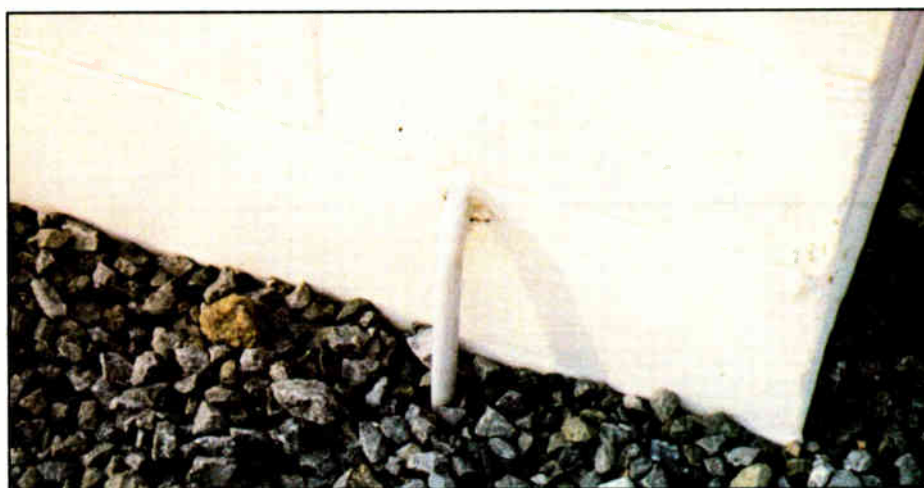
Figure 3: ... and exits the block building, protected by PVC conduit.
