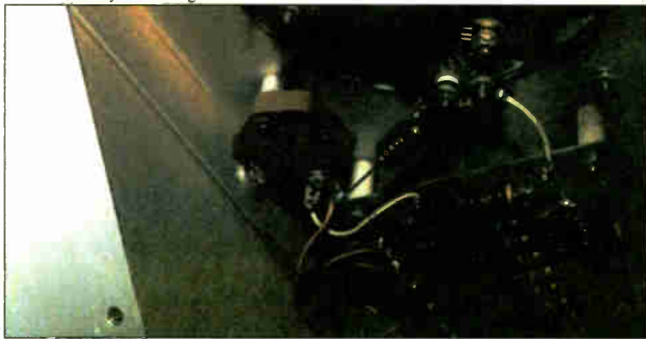
Figure 3: Check all wires for good, tight connections and intact insulation.
