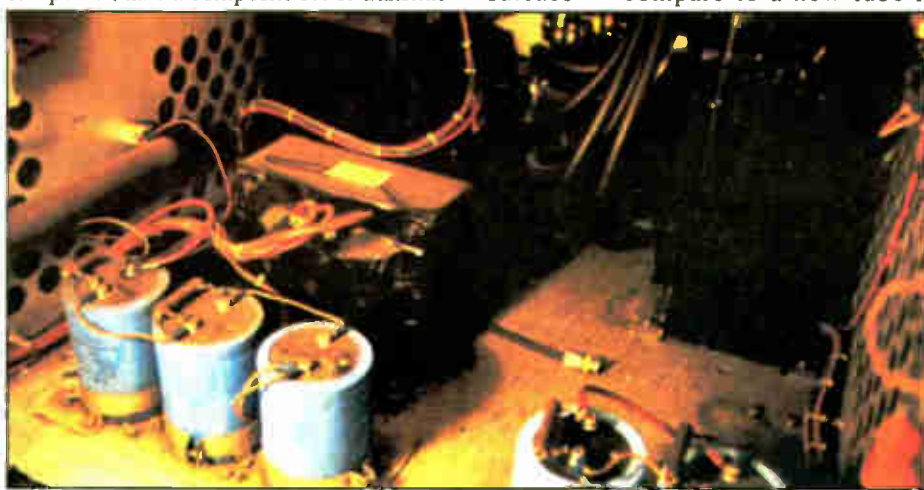
Figure 2: Keep the power supply vault clean.
