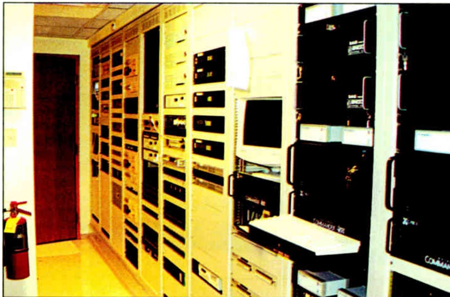
The Rack Room
