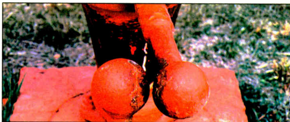
Figure 4: Clean spark gaps protect the coupling network. Carbon and pitting can be removed with crocus cloth.
