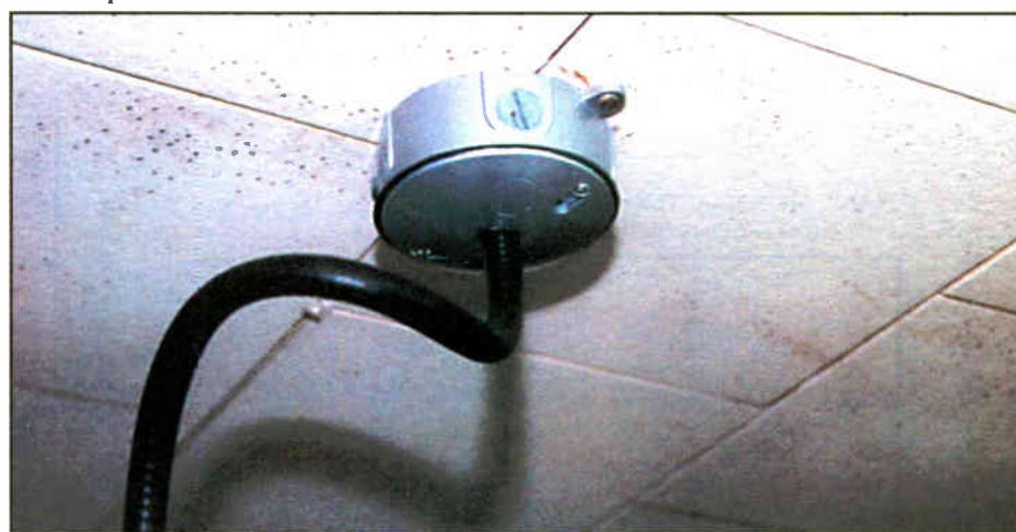
Figure 3: An electric box provides cable support and finishes the cable entry to the ceiling nicely.
