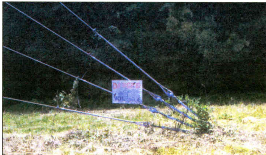
Figure 1: Keep vines and growth away from guy anchors to reduce maintenance headaches.
