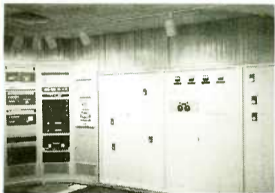
WIDEBAND DIRECTIONAL ANTENNA 50 / 5KW DA-2 PHASING SYSTEM WWRC-AM RADIO GREATER MEDIA WASHINGTON, DC
