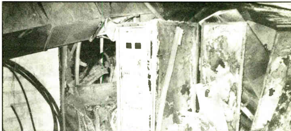
The fire left only debris and the charred remains of two 25 kW Continental transmitters.
