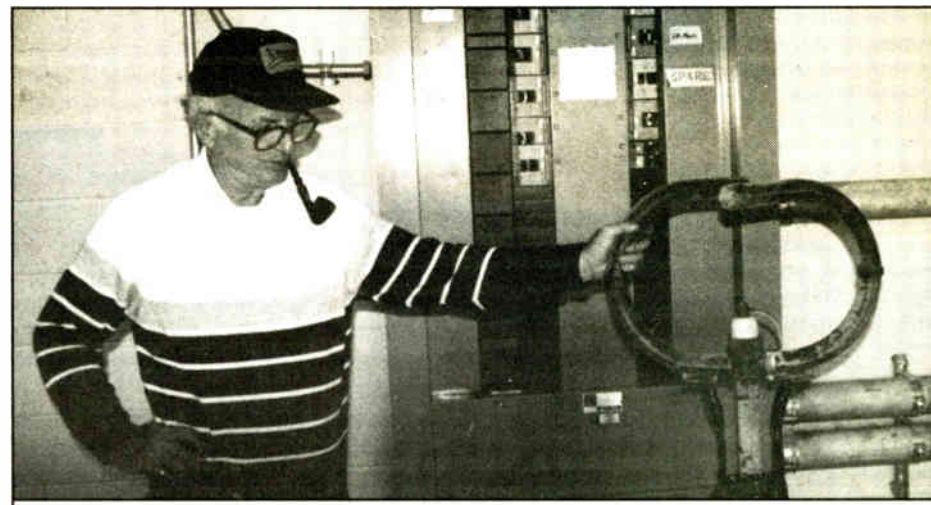
WRXL station engineer George Oberto stands by an antenna bay as it is repaired.
