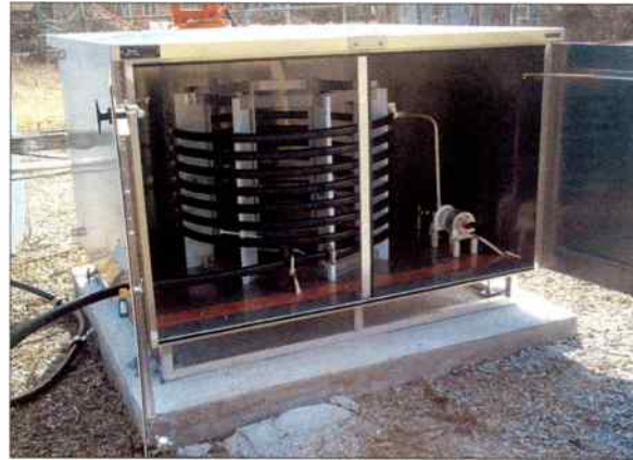
Kintronics Isolation Box
