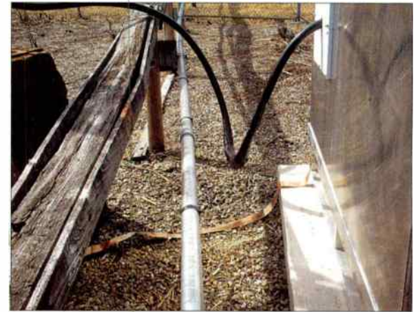
Burned, and Now Spliced Cable
