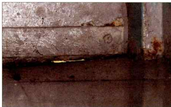
A crack found during a lights out inspection. This is an easy entrance for a field mouse and blowing cold air. The fix? A new door sweep cost $5.
