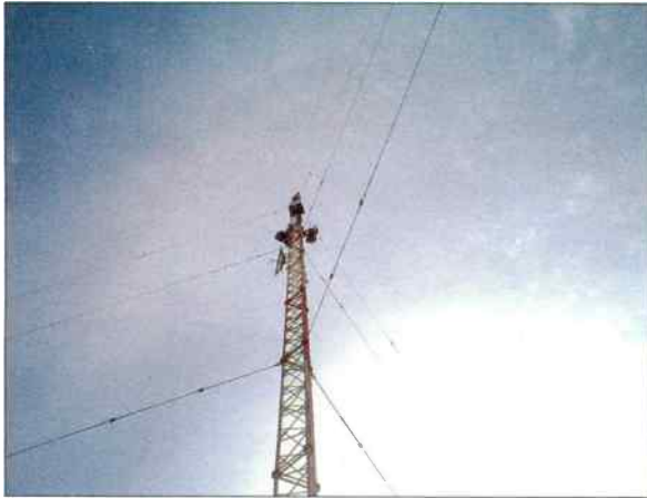
Cell-site Radios on Tower
