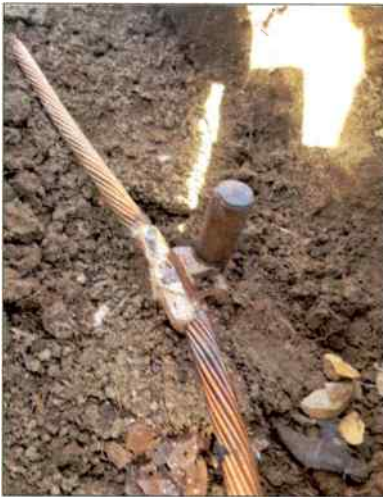
4/0 Cable Thermo Welded to Ground Rod
