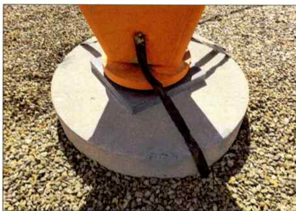
Original Ground Strap With No Ground Rods
