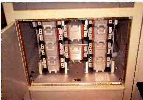
After output filter removal.
