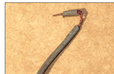
#10 copper wire reduced to copper thread by extreme corrosion.
