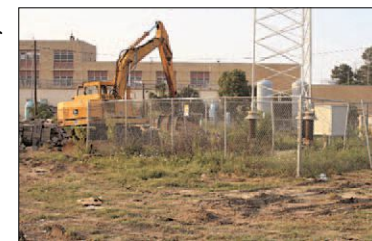
Exactly why is that trackhoe 20 feet from my tower?
