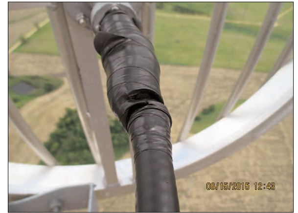
The antenna jumper had been damaged.
