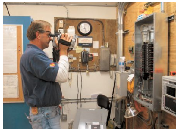
Mike Bivens of Infrared Services, Inc. views the breaker box with an infrared camera.
