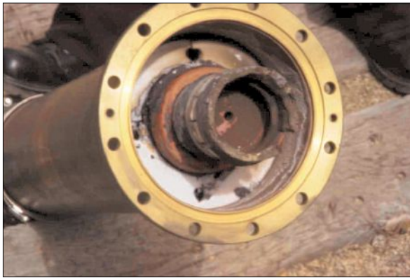
The antenna transformer failure was apparent.
