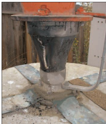
This is an ex-insulator.
