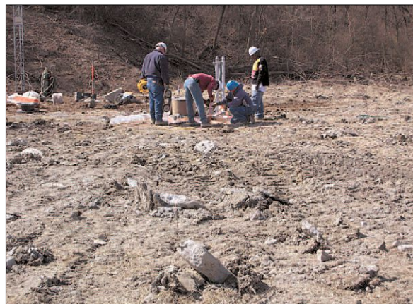
Concrete waste provided challenges.
