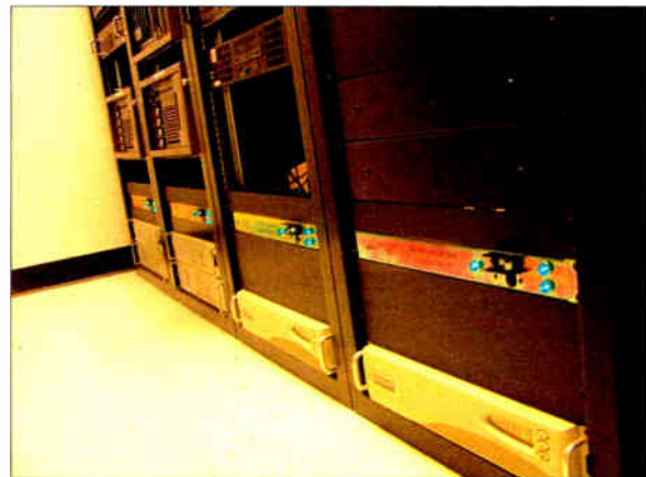
A server room at Entercom Seattle showing four UPS's (two different types) and automatic transfer switches.
