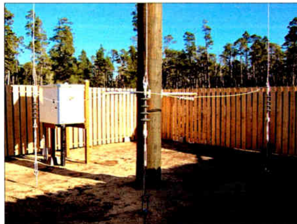
The feed point at the base of the center pole of the Kinstar antenna showing three of the four insulated vertical elements with the associated commoning ring.
