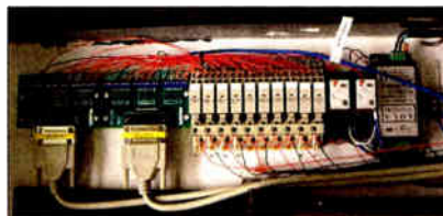
Building a breakout on a DIN ISO rail.
