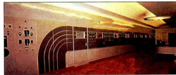
The 600 kW Aspidistra transmitter.
