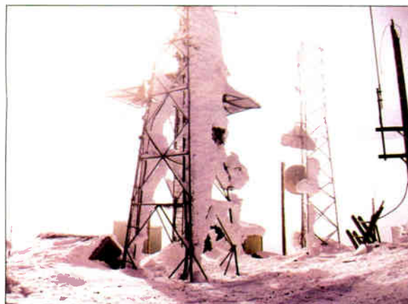
Snow and icing of the antennas are obvious issues.
