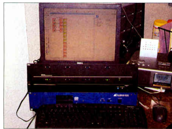
The Relio unit sits between the relay panel and the Audemat RDS unit at Wyoming Public Radio.
