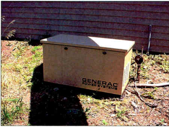
A home-sized generator will provide enough power to get something on the air.
