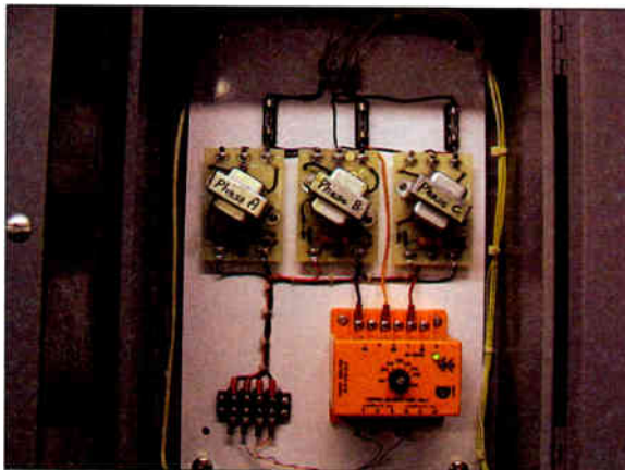
Inside Clay’s power monitor box.
