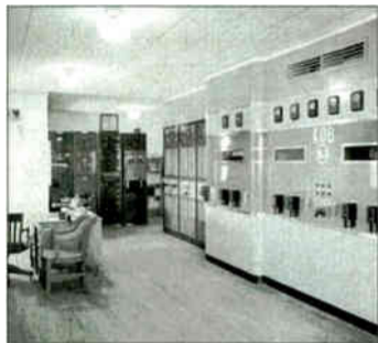
Inside the KOB transmitter room.
