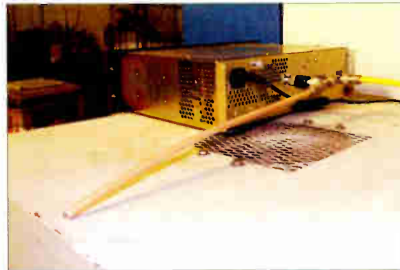
The stub attached to the back of the exciter. Note, too, the 3 dB pad between the exciter and the tee.
