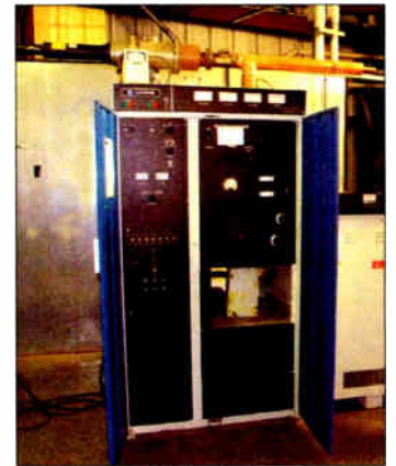
A working FM-20K is used for testing the rebuilt 4CX15000A tubes under real operating conditions.
