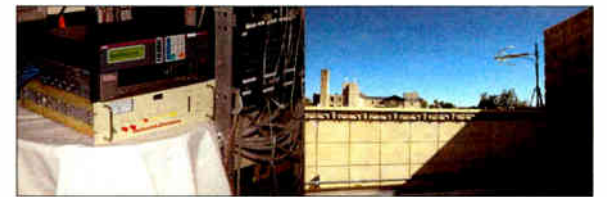
The KANA transmission system was set up close to the roof.
