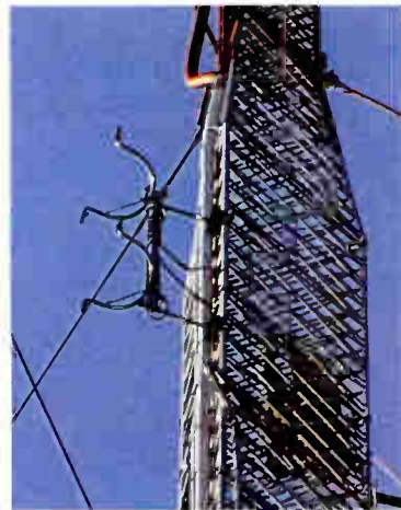
The JLST antenna mounted on the tower.
