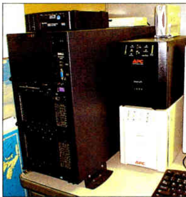
A dual power supply server with two UPSs
