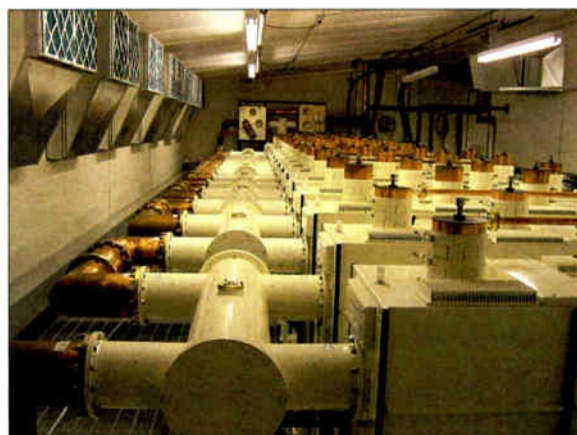
A 16-station combiner at Cougar Mountain in Seattle, WA.
