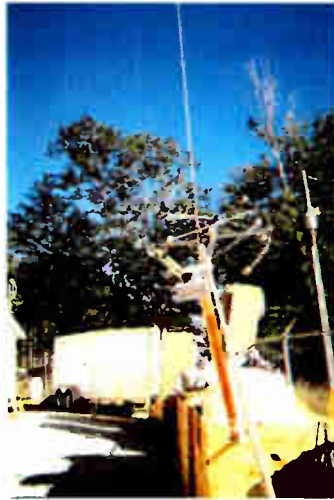
Up she goes! A bay of the Dielectric antenna is ready for installation.
