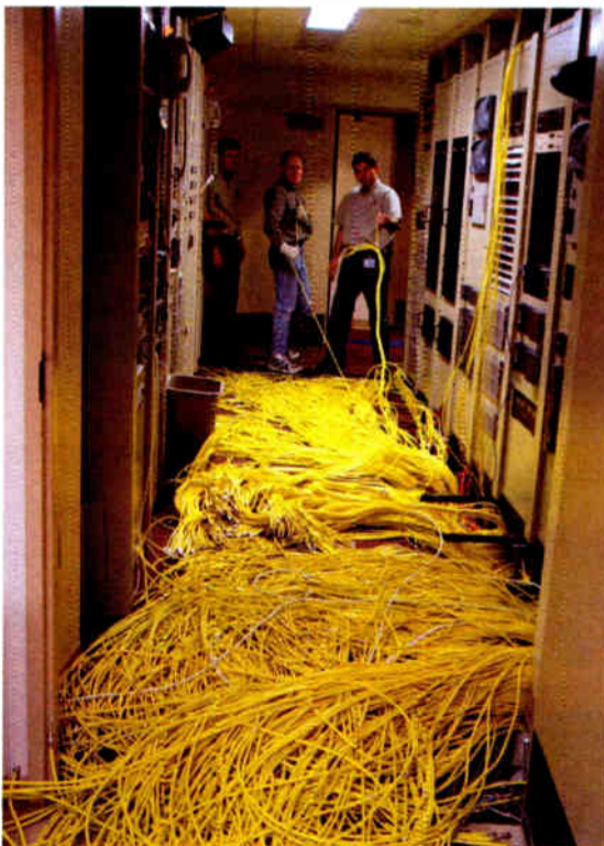
Pictured left to right: Gary Burgess, Engineer; David Gabbitas, TOC Engineer; Bob Wood, Engineer; and a whole lot of cable.
