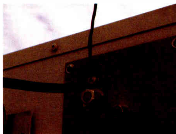
This feed point on the ATU is rusting and corroding, resulting in poor electrical connection.
