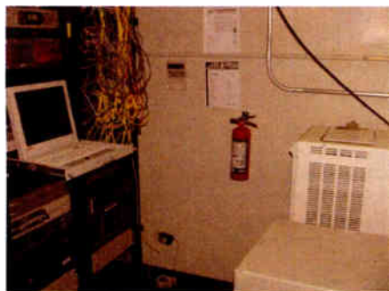
An Halotron I extinguisher stands guard in the rack room of a station. It is important to use the right kind of extinguishing agent.
