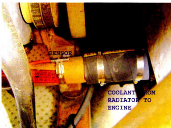
The second sensor is clamped to metal radiator outlet pipe.
