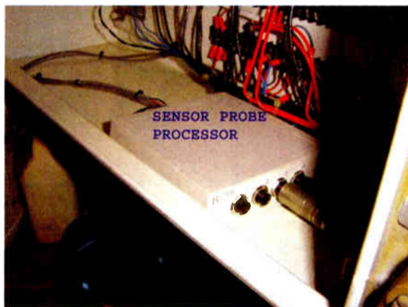
The temperature probes are connected to the Burk processor, installed in Louver control box.
