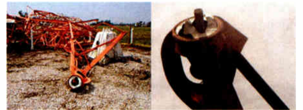
The insulators proved to be a weak point
