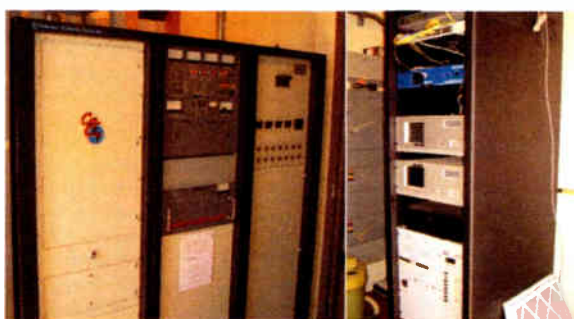
With high level combining, the HD rack, including IP connections.
