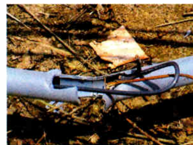
The schedule 40 conduit was torn apart and the entire DA control system was ravaged.
