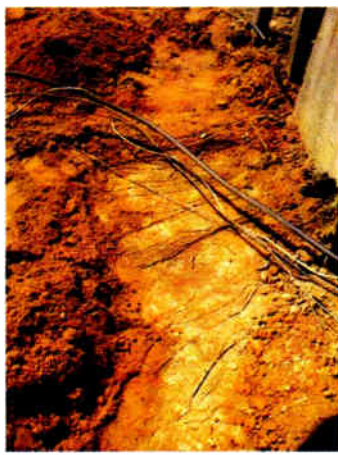
Vandals excavated around this tower base to remove copper sheeting.
