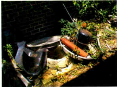
What was left of the HVAC units at the site.
