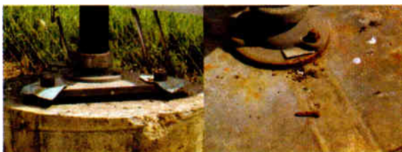
All the straps were cut right at the tower base, severing the tower from the ground system.
