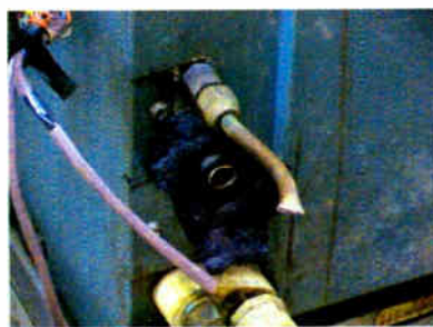
Even the copper tubing on the air conditioner was cut and stolen.
