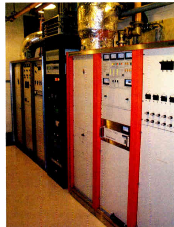
KRQQ's 816HD transmitter alongside the 816R-3 (now the Backup).
