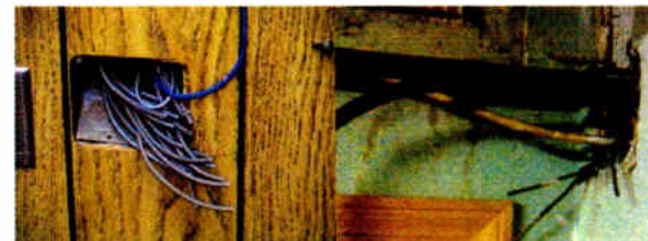
The station's coax, audio and control wiring were randomly cut.
