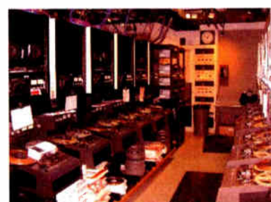
One of the tape rooms.
