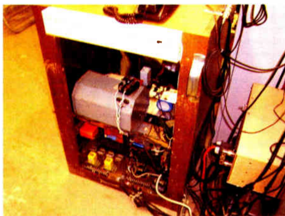
A curious transformer and a lot of "stuff" hiding in a rack.
