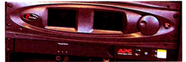
With many transmitters having computers as their core, UPS is a necessity.
