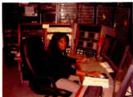
Master Control Operator Donna Harrell monitoring 13 separate on-air audio feeds. The operating desk is capable of controlling 100 separate programs
