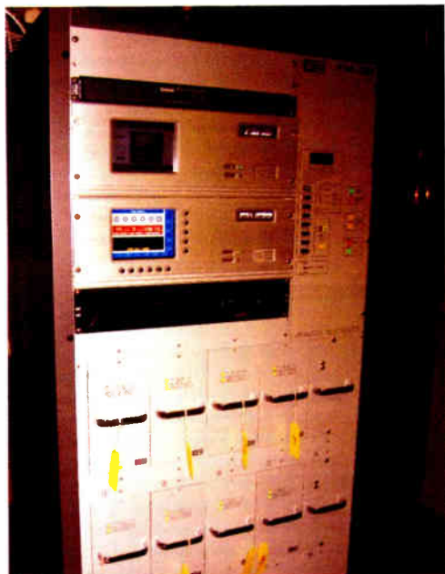
BE FMi 301 installed in WLTW transmitter room.
