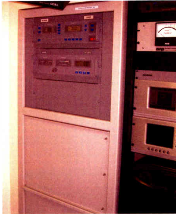
One of the four Harris Z10s in the WHTZ/WKTU transmitter room
