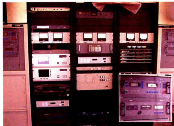
WKTU Equipment racks and Z10CD transmitter.
