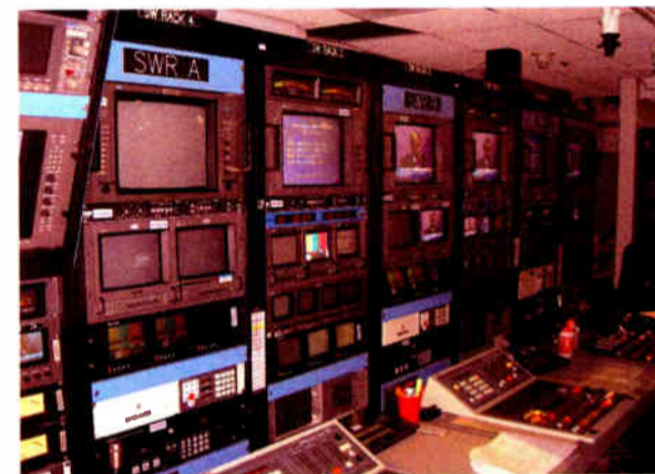
A small portion of the television transmission control room.
