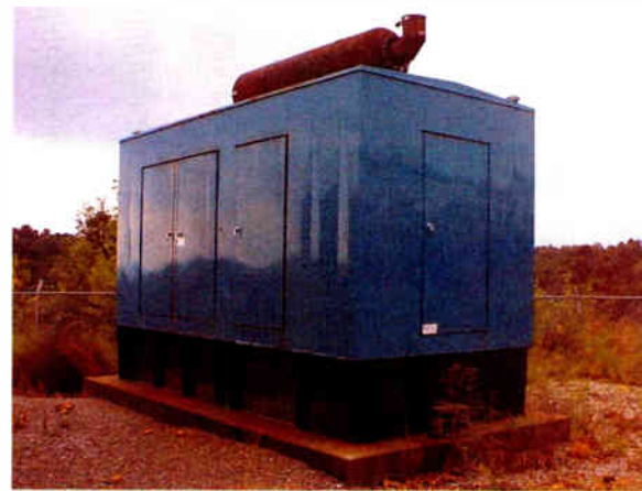
WKBI's large 800 kW Generator. Note the cinderblock needed to reach the door.
