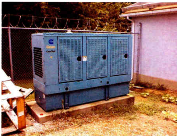
A modest-sized generator for broadcast use.
