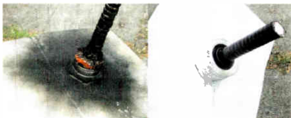
Left: Cable Penetration Flame Side, with extensive damage.
