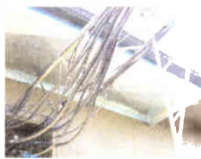
Roof Fire Shield
