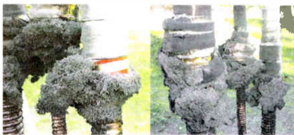
Burned Cable and Activated Fire-Stop
