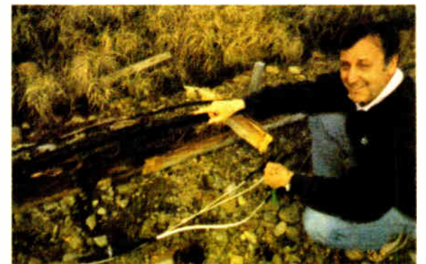
Dennis Weidler, GM of KICY AM/FM, Nome AK, showing damage to transmission coax.
