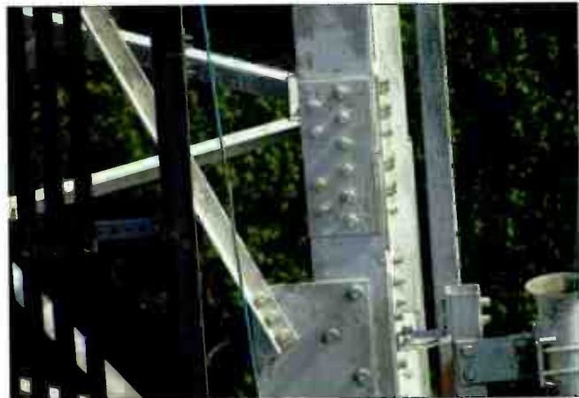
High-resolution photographs taken from a safe distance of 15 to 30 feet from the Willis tower allow examination of hanging cables and tower bolts.
