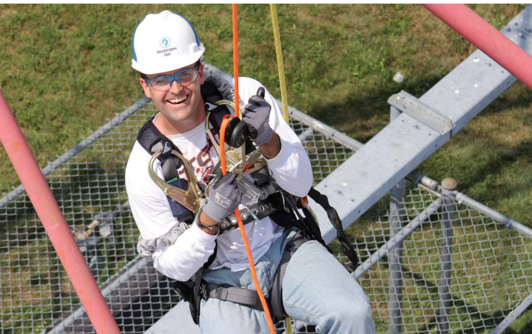
Todd Schlekeway, executive director of the National Association of Tower Erectors, descends from the tower using a controlled-descent device. "We wanted to demonstrate leadership in participating in the course from beginning to end. We're putting our money where our mouth is," he said. Photo by Rusty Datman
