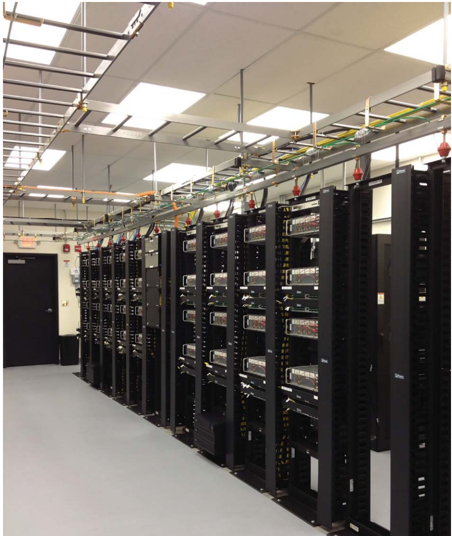
This is the head end for the Churchill Downs upgraded distributed antenna system, which is designed to support the yearly attendance at the Kentucky Derby and the anticipated continuing increase in mobile network traffic.
