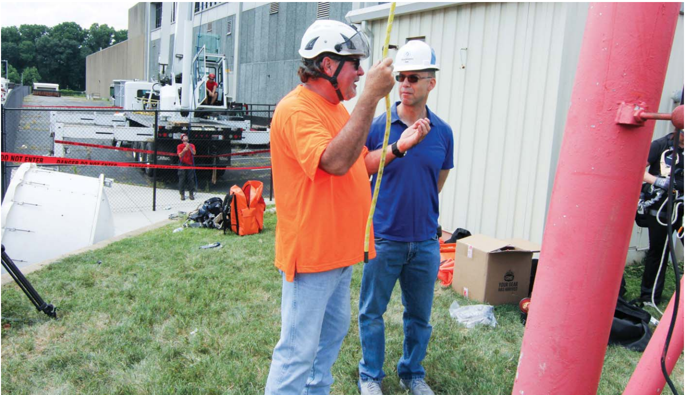
With the crane operating in the background, John Paul Jones, vice president of training at Safety LMS (left), speaks with Jonathan Adelstein, president and CEO of PCIA, who paid a visit to the Washington Gas tower site on July 22. "It's great to see that a lot of people in the industry are learning how to climb, safety, and basic techniques so when it comes to training others and ensuring safety, they have firsthand experience of how it actually works," Adelstein said. Photo by Rusty Oatman
