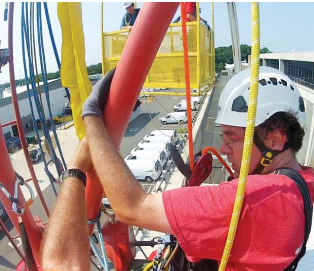
The personnel basket manned by Jim Goldwater and Zach Johnson approaches. Schlekeway is at a level below Rich Biby (foreground), and his harness is attached to Biby's. Biby will swing Schlekeway over to the basket.
