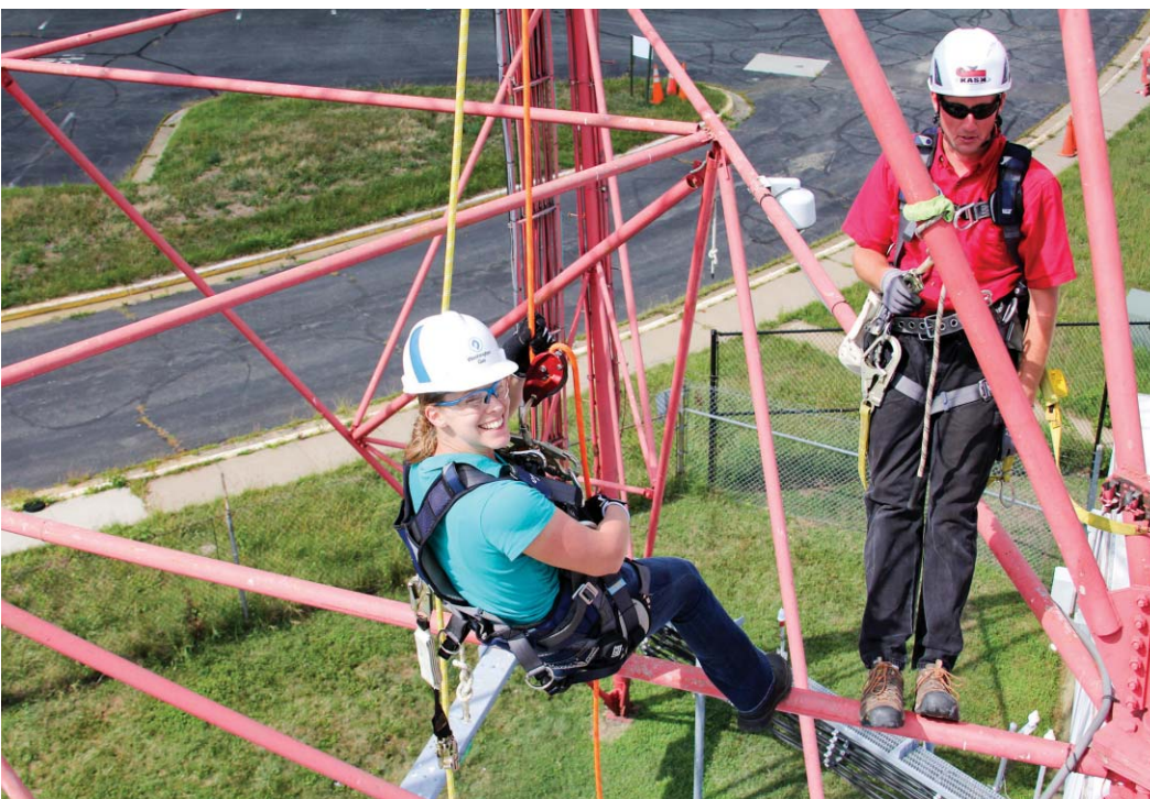
As Zach Johnson, safety and training director at Shenandoah Tower Service, looks on, Jessica Douma, a regulatory analyst in the OSHA Directorate of Construction, prepares to descend. She is using a controlled descent device on the red rope while connected with fall-arrest apparatus on the yellow rope. Photo by Rusty Oatman
