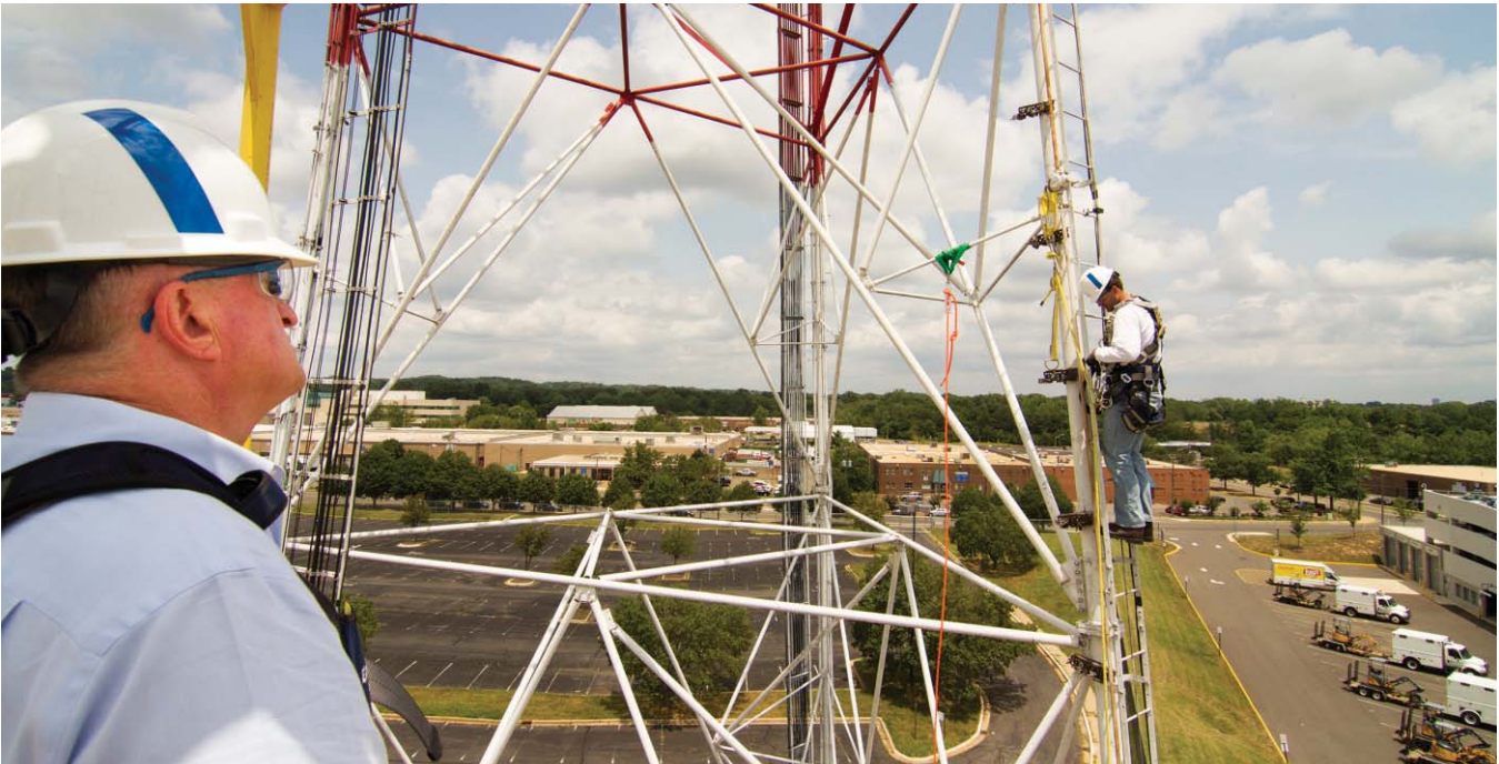
From the vantage point of the personnel basket held at height by a crane, Gordon Lyman looks over at Todd Schlekeway as he pauses during his ascent of the tower on the first day of training at the structure. Photo by Don Bishop
