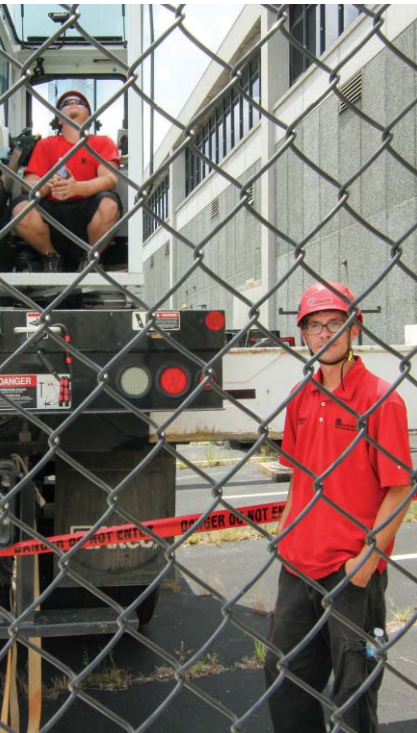
Eric Severs from Shenandoah Tower Service operated the crane. Brandan Hardy monitored the crane and personnel basket, keeping people away from the area beneath the basket. Photo by Rusty Oatman
