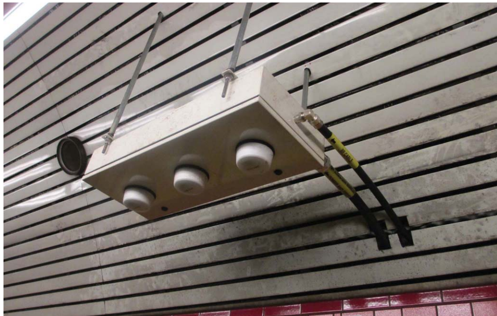
The access point box is a 36-inch-by-50-inch box that houses all the Wi-Fi equipment and the switch. It is where the three MIMO antennas are placed. The heat dissipation is through the walls of the equipment box itself.
